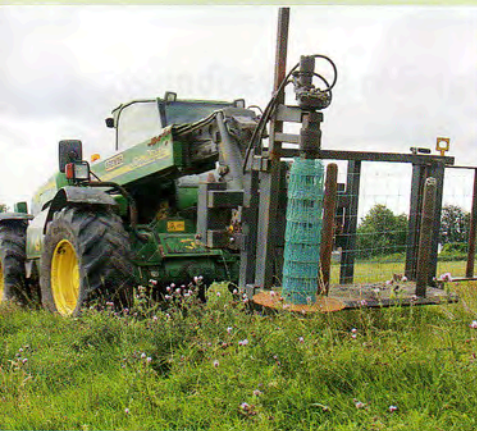
The wire builds up on the roller as it is rewound using the hydraulic motor mounted on the top.
