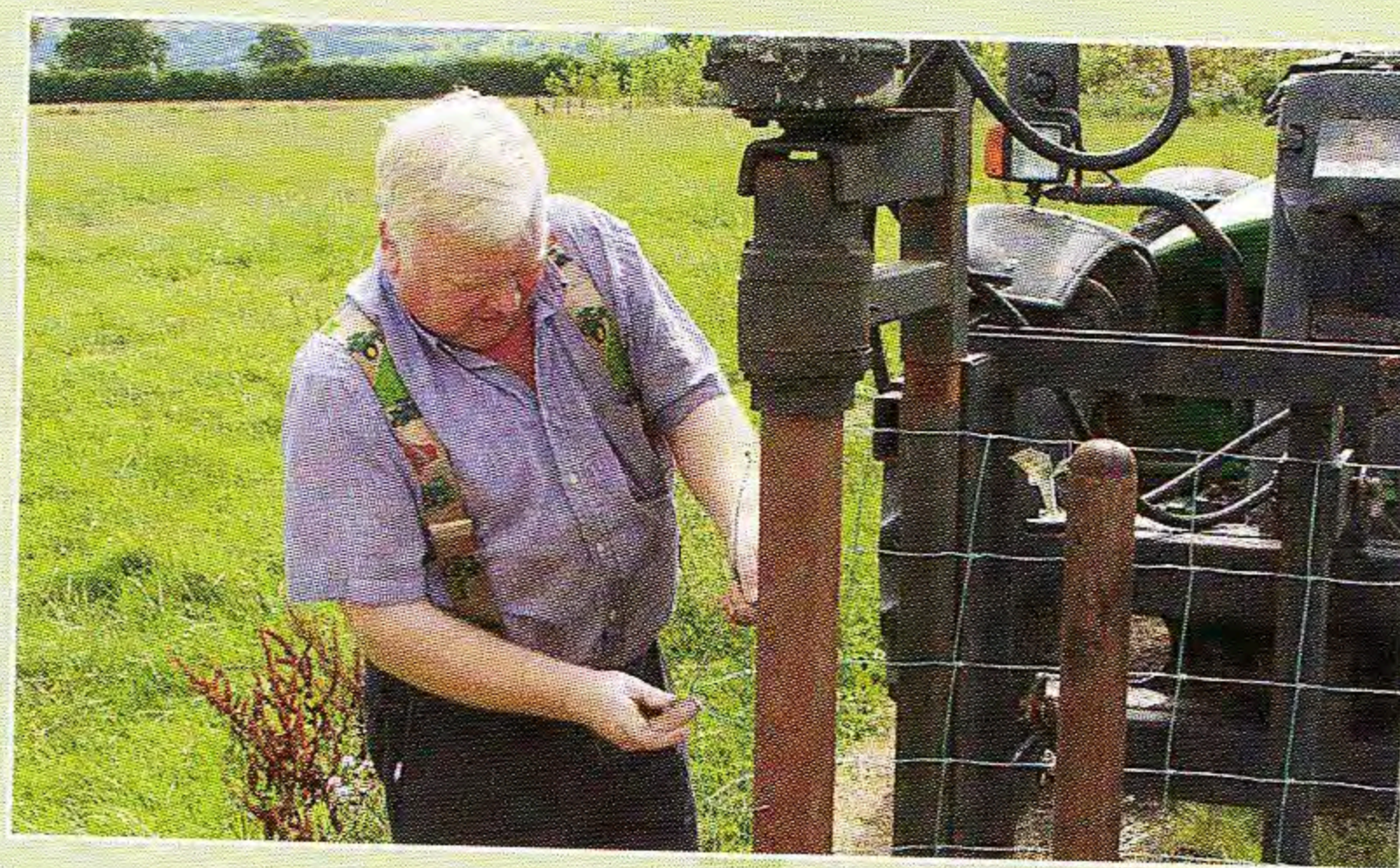
If the fence is only temporary, the wire can be rewound using a hydraulic motor. Mr. Brewer attaches the wire to the rewind roller.
